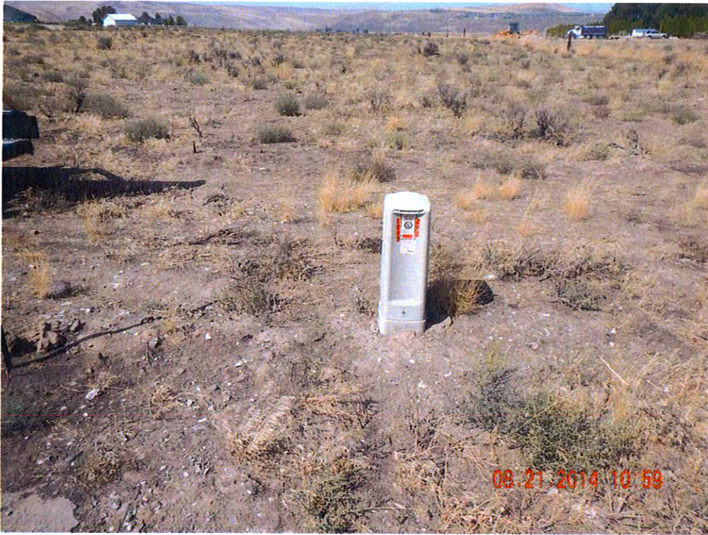
9. Telco Pedestal south of the southwest corner of the host parcel.
